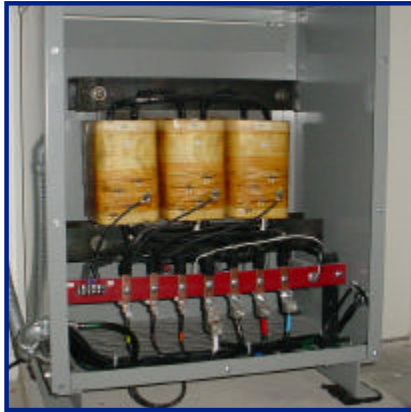
Zero Sequence, Harmonic Mitigating Transformer by Olsun Electrics installed at the San Antonio International Airport.
